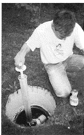
Access risers to grade and an effluent filter have been installed on this septic tank. These two simple retrofits allow for ease of maintenance and help to prolong the life of your system.
