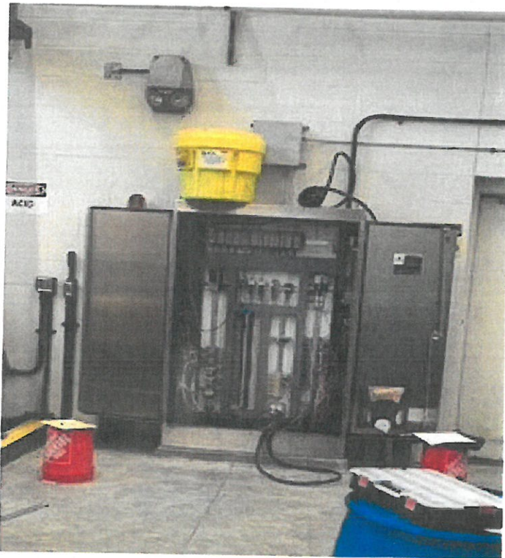
Cabinet with new process controls installed
