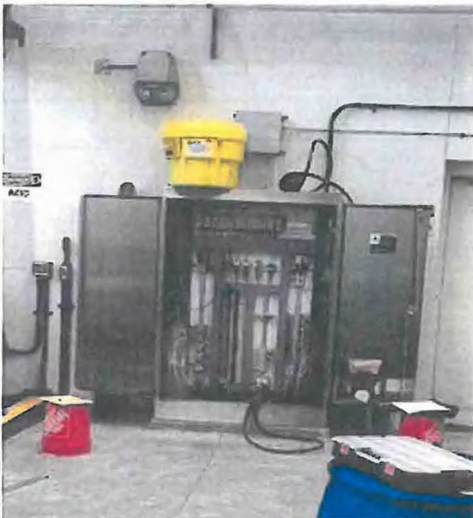
Cabinet with new process controls installed
