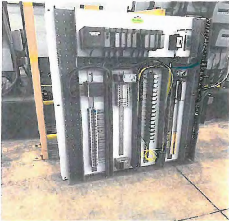
Existing process control board removed from cabinet for installation of new equipment
