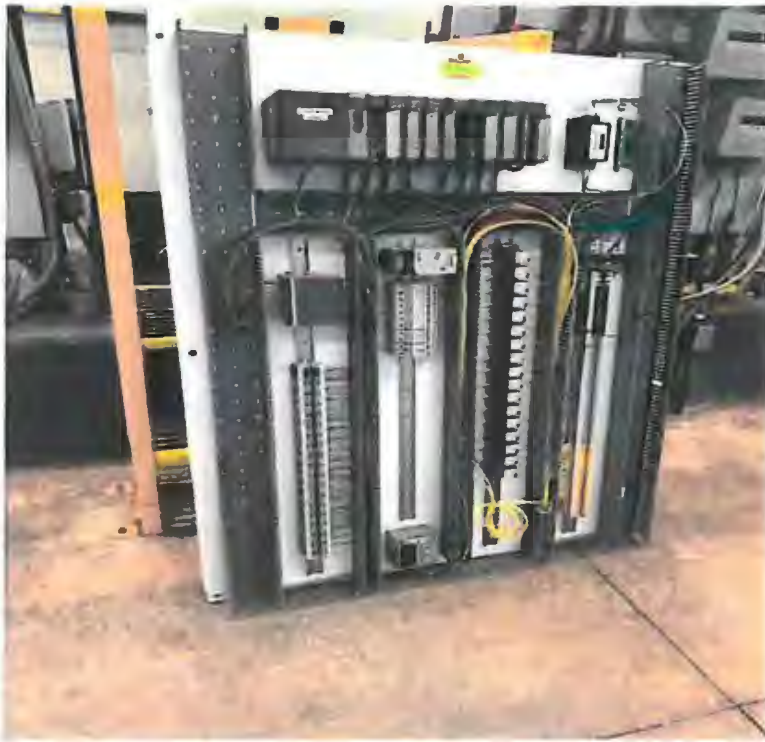
Existing process control board removed from cabinet for installation of new equipment
