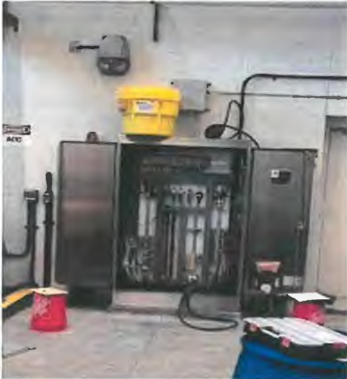
Cabinet with new process controls installed
