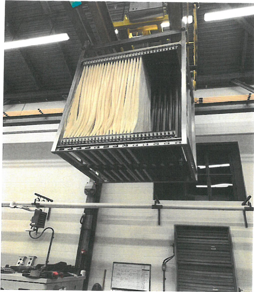
Old membrane filter ready for replacement
