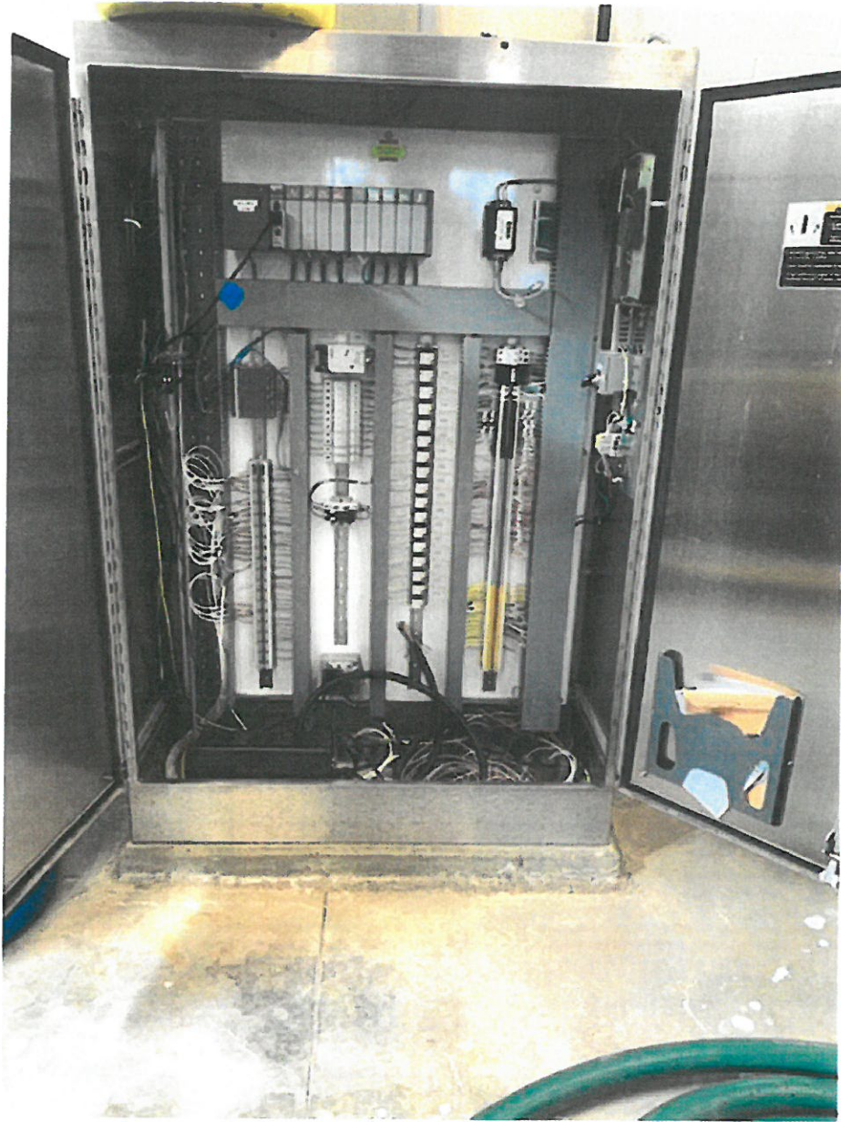
Control Equipment scheduled for replacement
