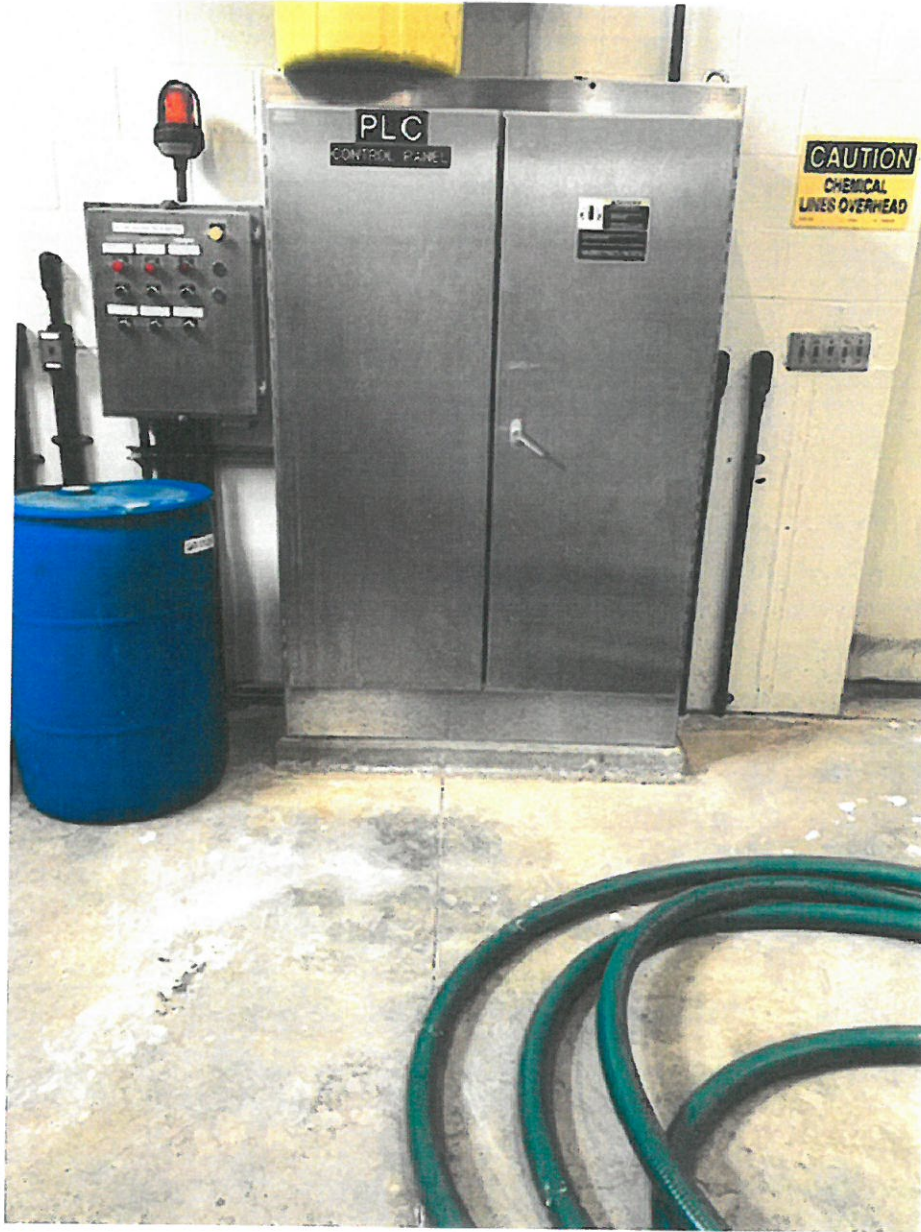
Program Logic Control (PLC) panel
