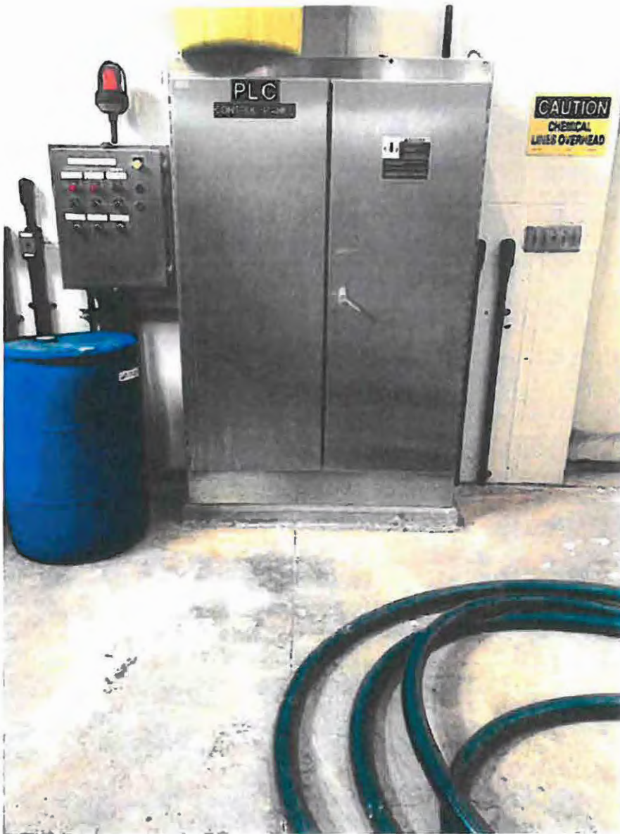
Program Logic Control (PLC) panel
