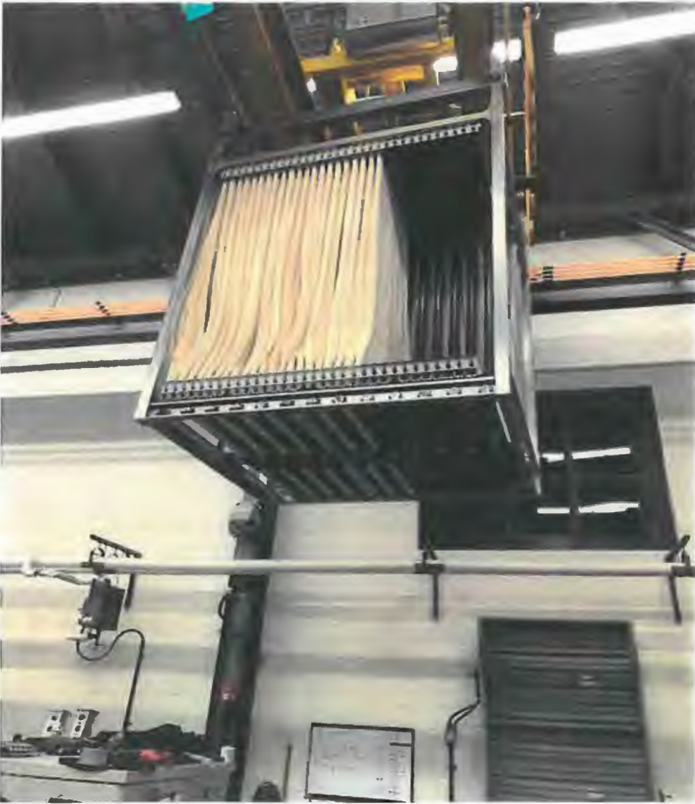
Old membrane filter ready for replacement
