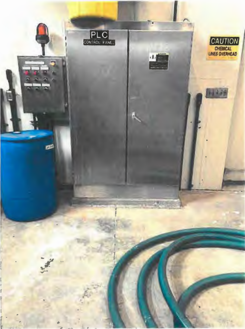
Program Logic Control (PLC) panel
