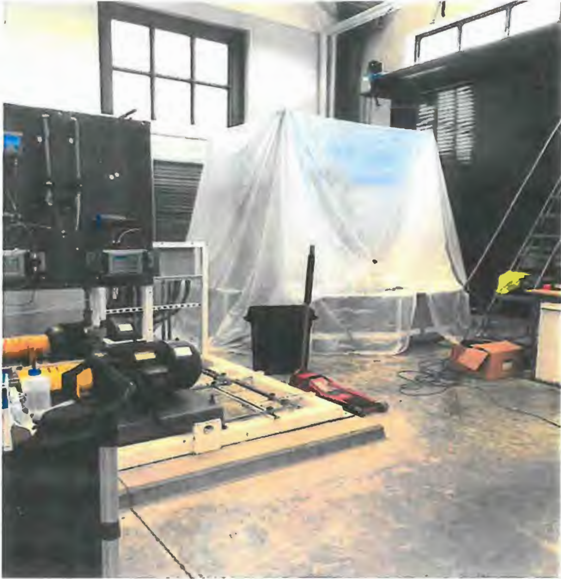
Filter for train one maintained in pool of water to keep membranes in a moist environment during tank coating
