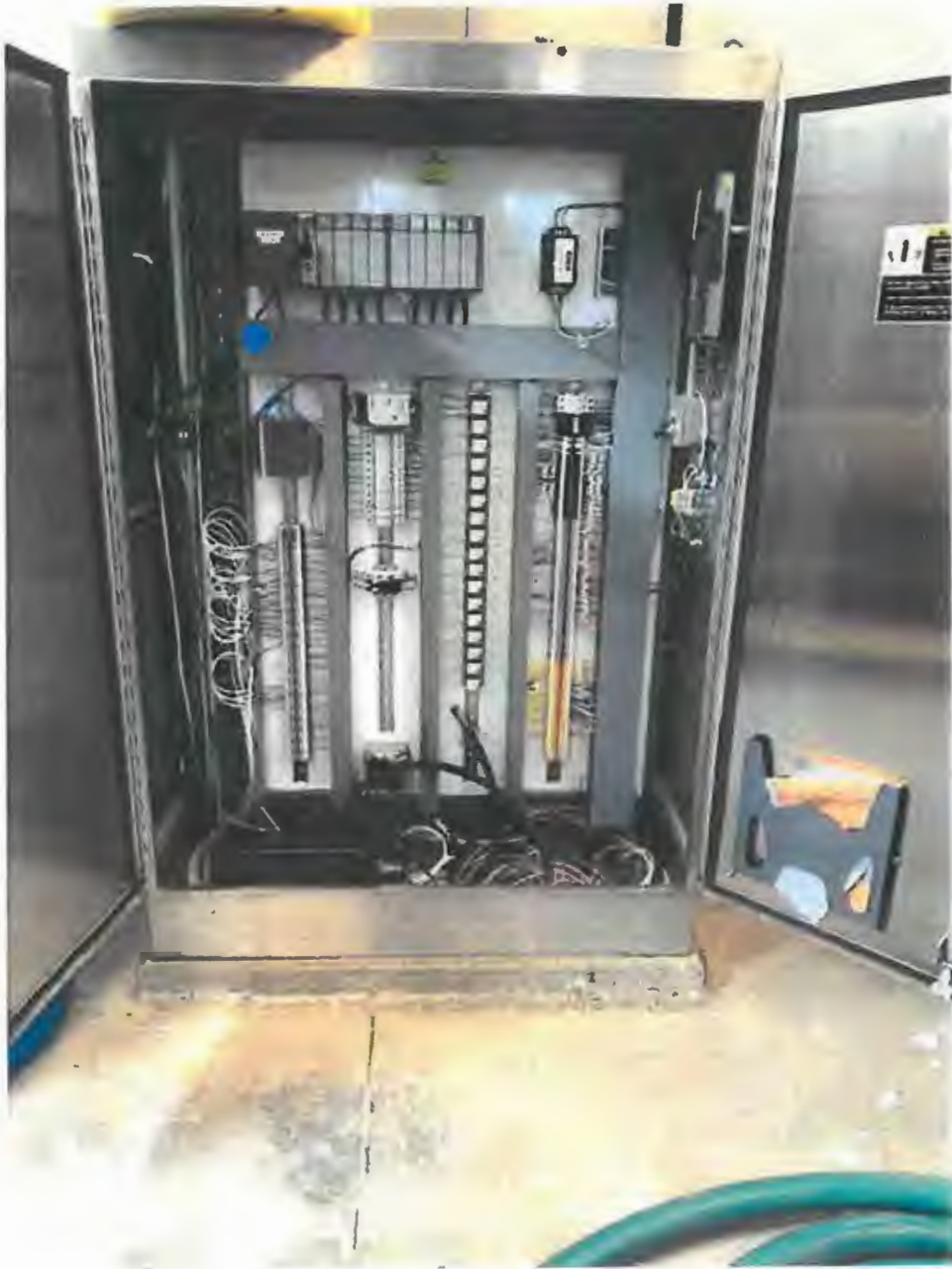
Control Equipment scheduled for replacement
