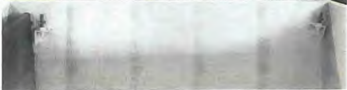
Tank for train one in foreground newly coated white. Tank for two still in use. Can see the difference in coating color and condition
