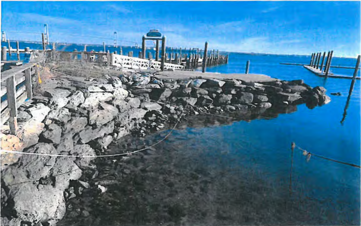
Photo looking East toward the Ferry Landing and the Wood pile pier in the background
