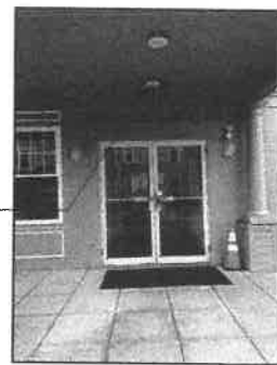
EXISTING EXTERIOR LIGHTS TO REMAIN
