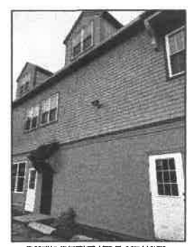
EXISTING EXTERIOR LED FLOOD LIGHTS TO REMAIN AT THREE LOCATIONS, TWO LIGHTS EAST ELEVATION, ONE LIGHT SOUTH ELEVATION.
