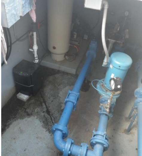
Tank Transfer Pump/Vault
