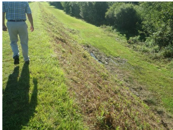
Seepage at Toe of North Pond Dam (looking east)
