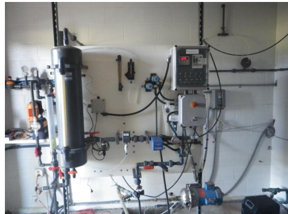
New Dosing Pumps
