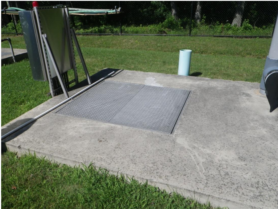
RAW WATER WET WELL
