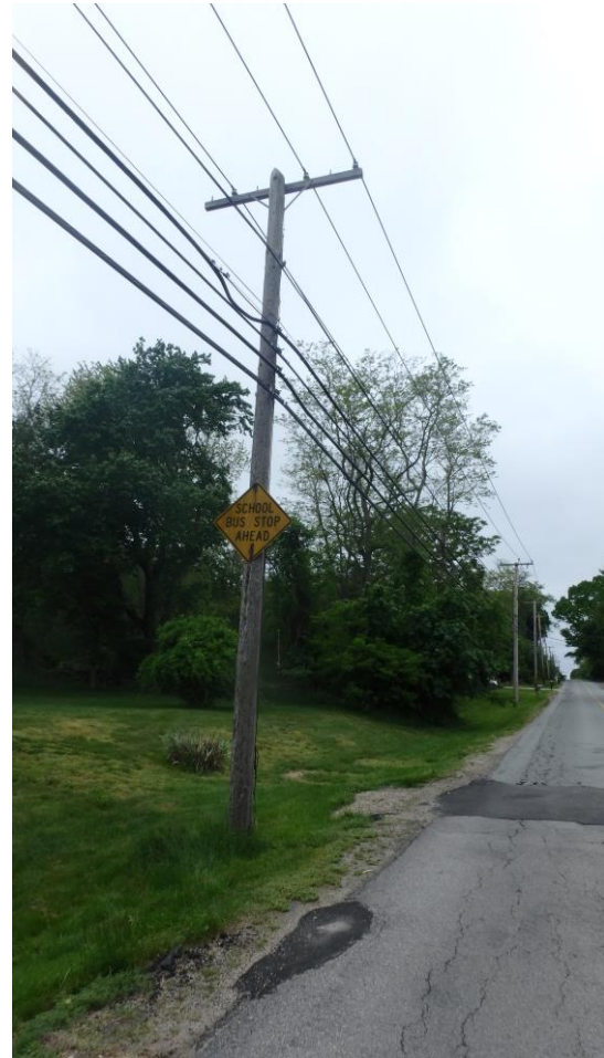
Utility Pole NET&T Co-110
