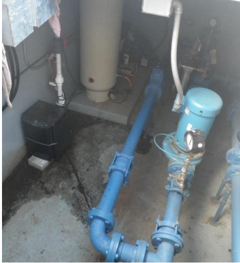
Tank Transfer Pump/Vault
