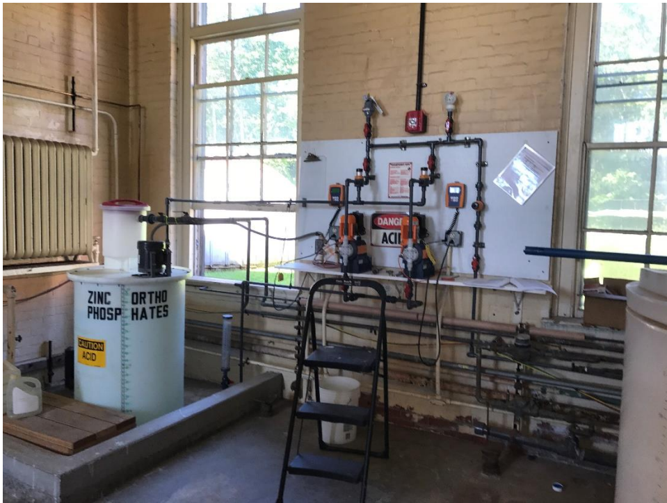
CHEMICAL MIXING – OLD TREATMENT BUILDING
