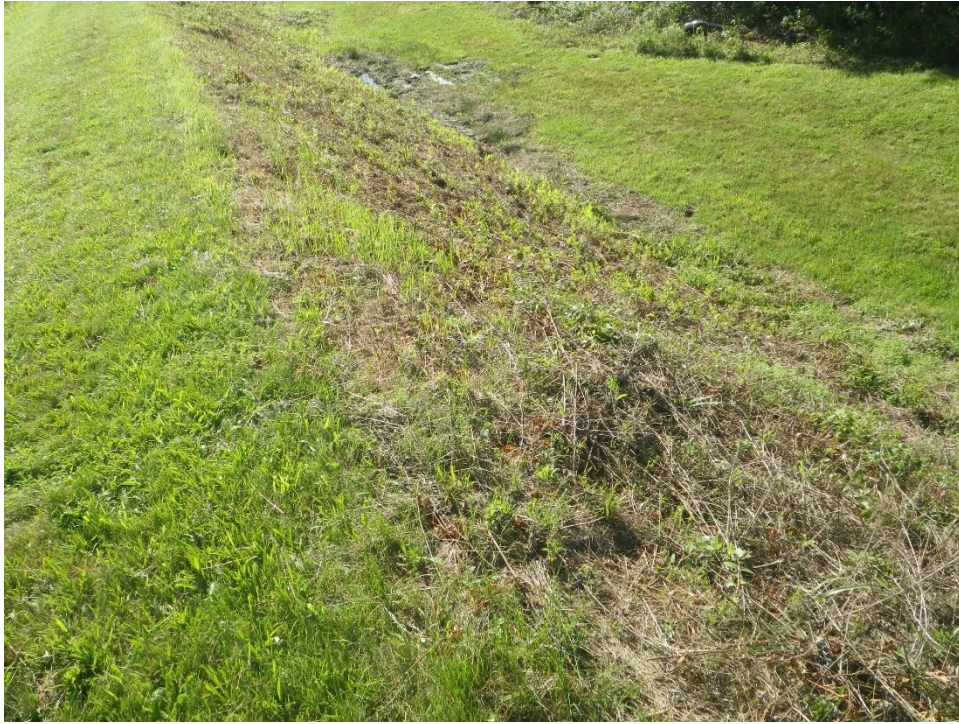
AREA OF NOTED SEEPAGE
