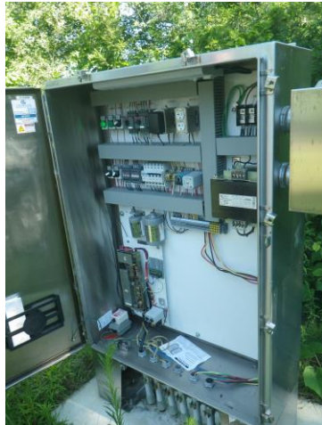
JR-1 Pump Control
