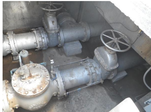
Standpipe #1 Altitude Valve
