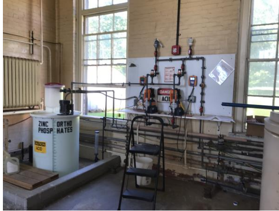
Old Treatment Plant Building Corrosion Control System
