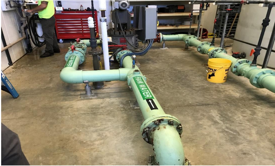
RAW WATER ENTERING BUILDING
