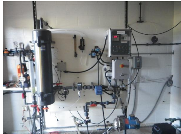
New Dosing Pumps
