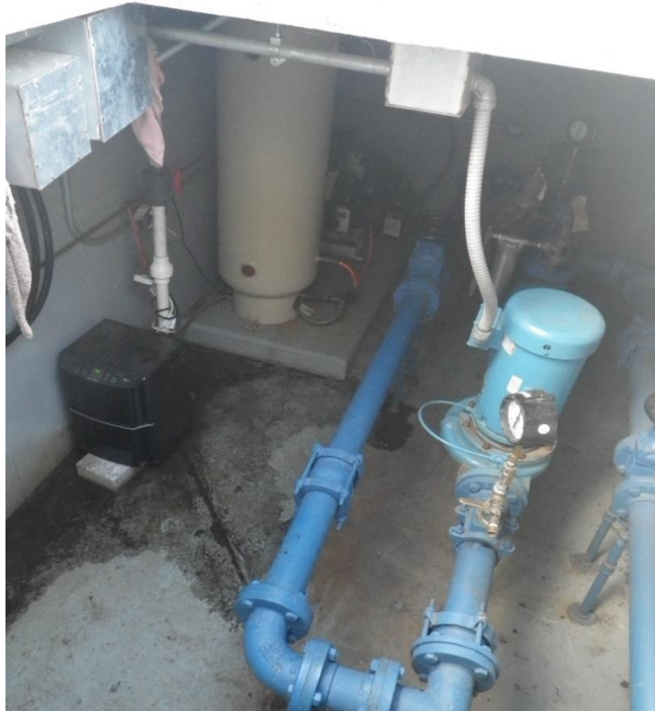
STANDPIPE TRANSFER PUMP
