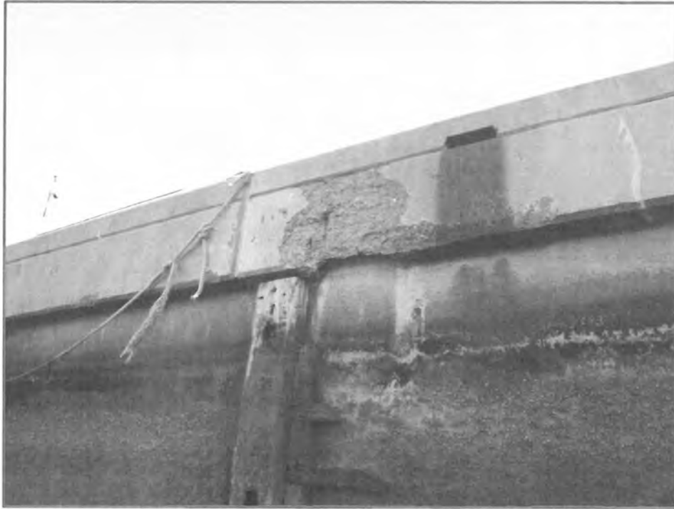
Photo No. 13: Concrete spalling along curb on North face of Pier, looking south, photo taken on March 23, 2019.
