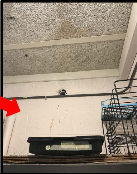
Teacher storage closet, with bin to catch leaking water.
