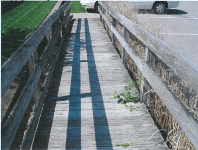
Maintenance required. Not in compliance with ADA
