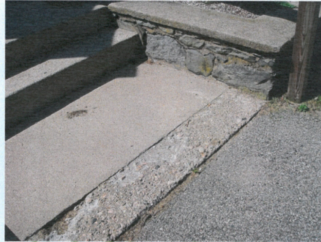
Paving corroding causing potential trip hazard
