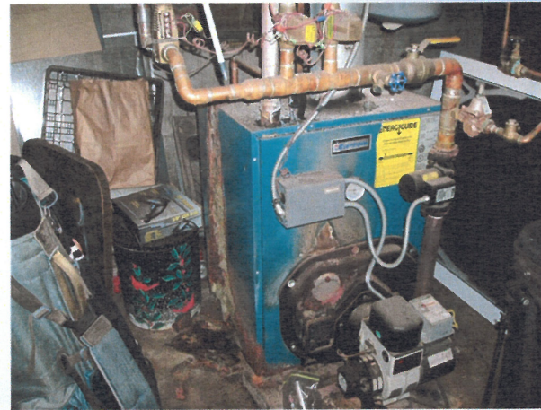
Current Heating Plant
