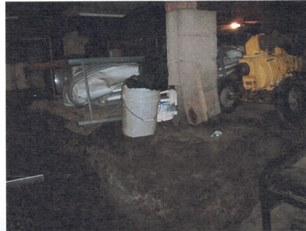
Unstable footings and support
