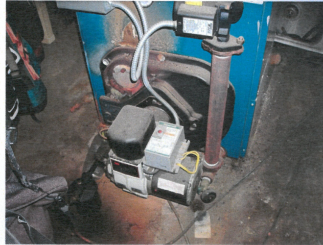
Corrosion at furnace
