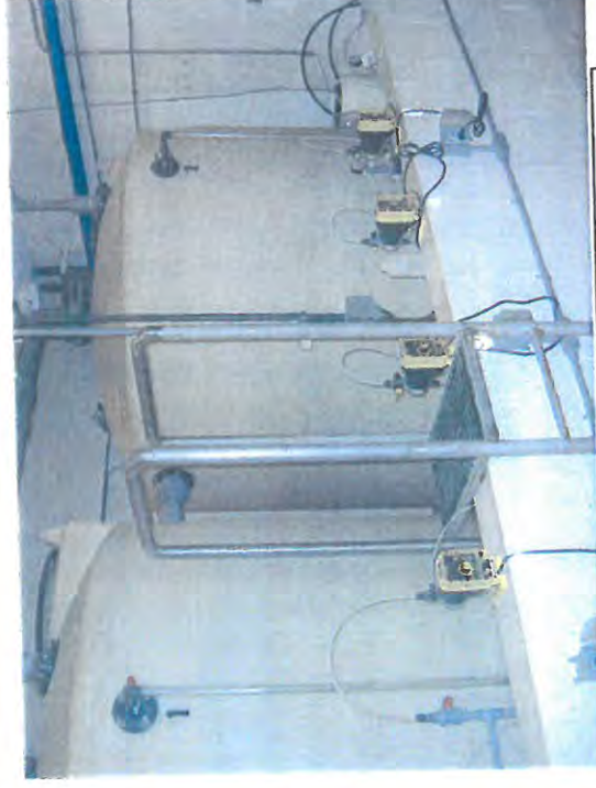
Above: Sodium Hypochlorite storage tanks. Tank #2 is not available due to a leak.
