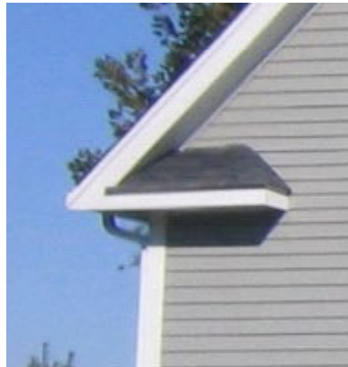
18.3 Discouraged. Eave return is much too long - extending further past the corner board than it should. The pitch at the return significantly exceeds 1:12 - probably more like 8:12 in this case.
