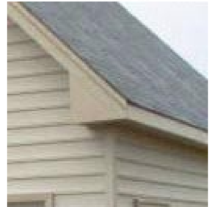
18.4 Unacceptable. The ubiquitous "pork-chop" eave return avoids the issue of the pitch at the return by fully enclosing the eave in a triangular "box" at the intersection of the eave and rake.
