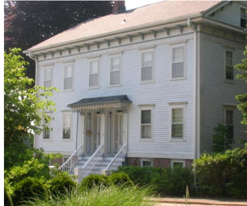
6.2 One simple gable roof is all that is necessary to shed water from this large duplex.
